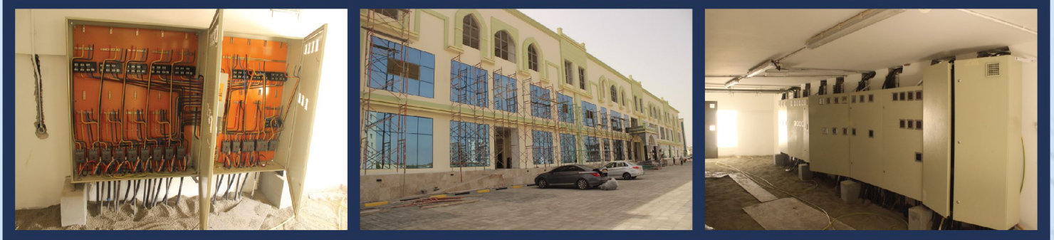
Commercial & Residential Building, Al Khoud Client : Shk. Salim Muslem Al Qatani Scope Description : Complete MEP installation and ELV System.
